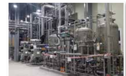
CO 2 liquefaction plant - Korea 200S / 230kW
