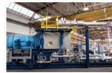
PSA compressor - Russia 400L / 1320kW
