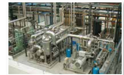
NH 3 recovery / Purification plant - China 2520SSC / 280kW
